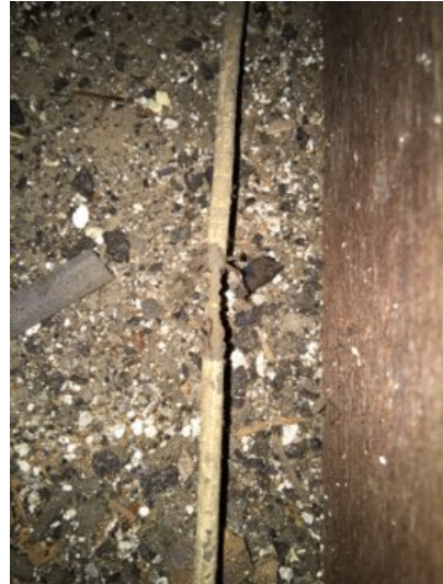
Deteriorated sheathing observed, see photo.
