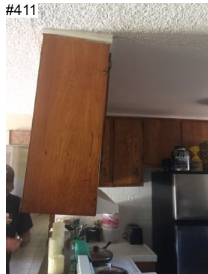
Noted cabinet(s) separating at the ceiling. Recommend having a qualified contractor re-fasten the cabinets. #411
