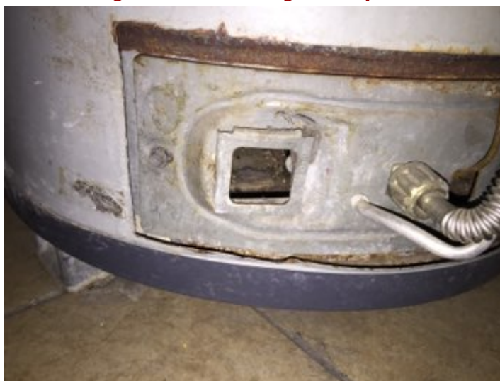
Chamber glass is missing. See photo
