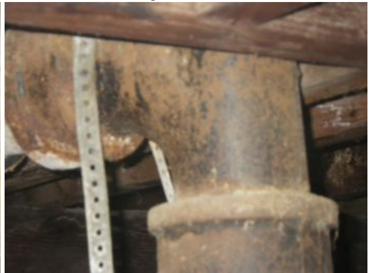
Cast iron drain lines have a life expectancy of 30-50 years. Recommend budgeting for replacement in the near future at areas where rust cysts are visible, BEFORE leaks occur.
