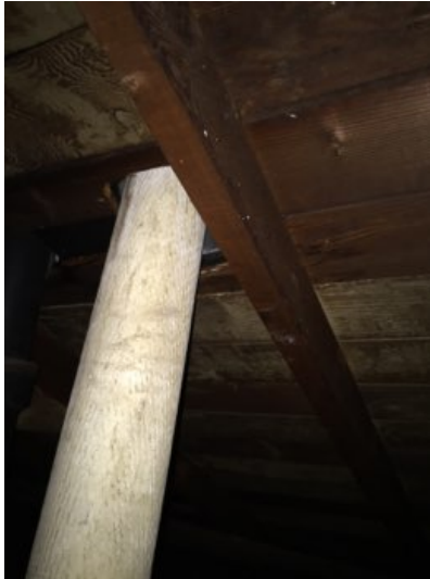
Transite type exhaust pipe observed
