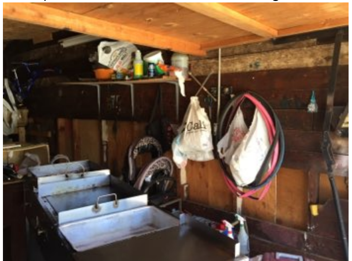
Personal items in garage block complete inspection of all floor, wall and ceiling areas.
