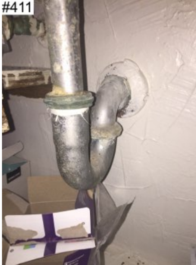
Older style metal traps noted. Buyer is cautioned that these traps can leak at any time due to corrosion.
