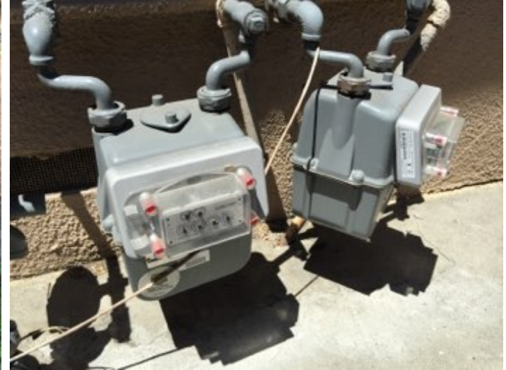
Meter located at exterior. All gas appliances have cut-off valves in line at each unit. No gas odors detected.
