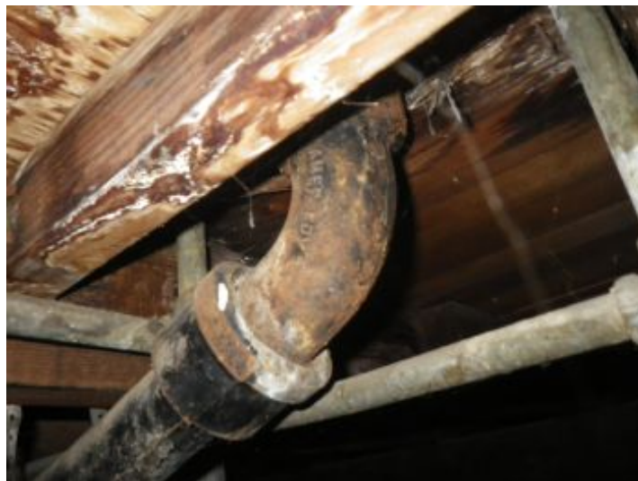
Wood rot, moisture damage observed. consult termite report
