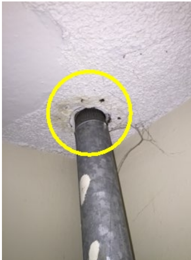
Loose connections noted.
