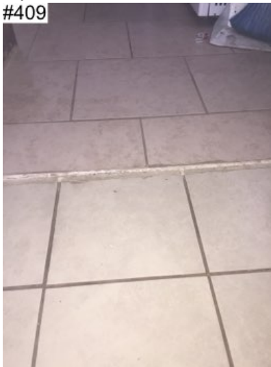
Missing threshold. This can be a trip hazard
