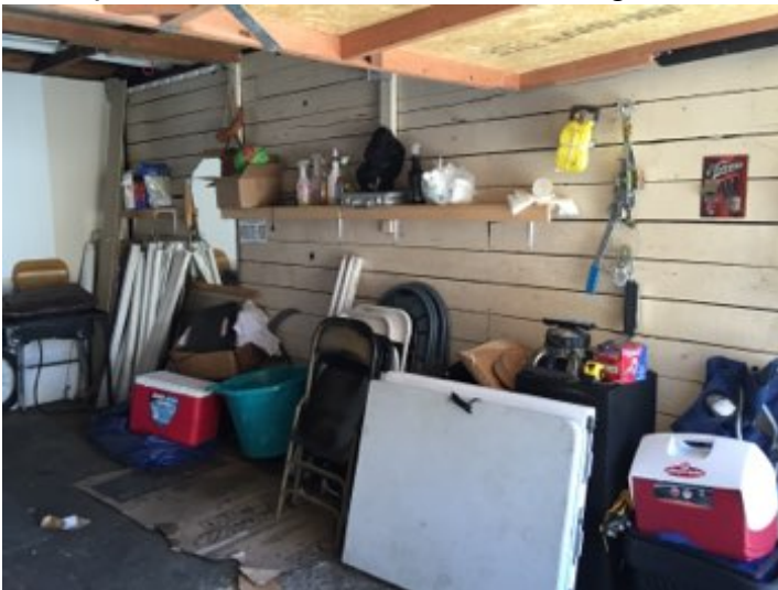
Personal items in garage block complete inspection of all floor, wall and ceiling areas.
