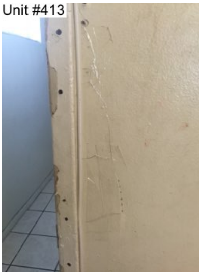
Damaged walls noted.
