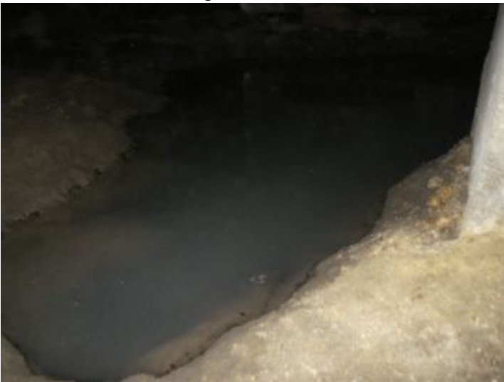
Standing water observed.
