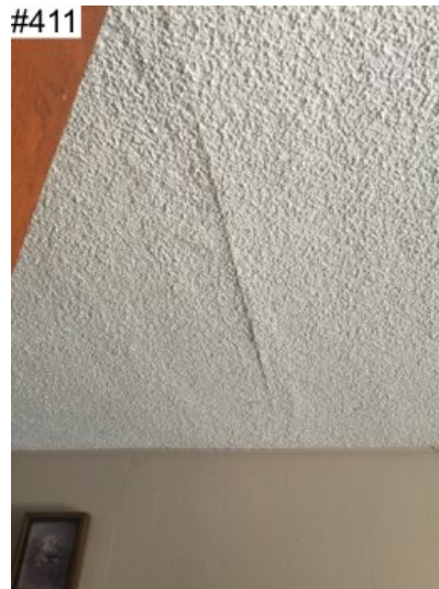
Settling cracks noted.
