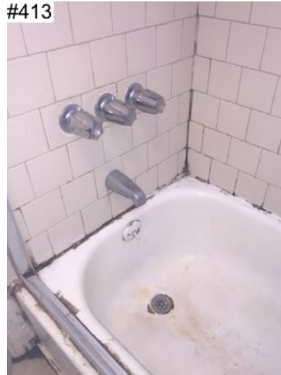
Caulking needed around perimeter.
