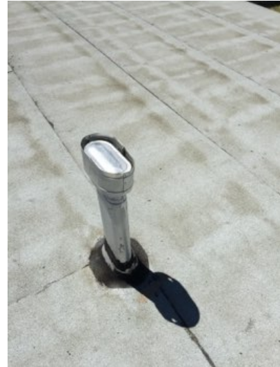
Note that experts recommend that any roof over 10 years old receive a roof certification by a local roofing specialist.
