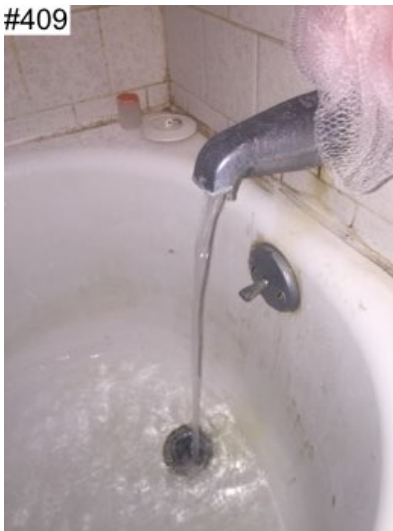
Shower diverter does not fully engage.
