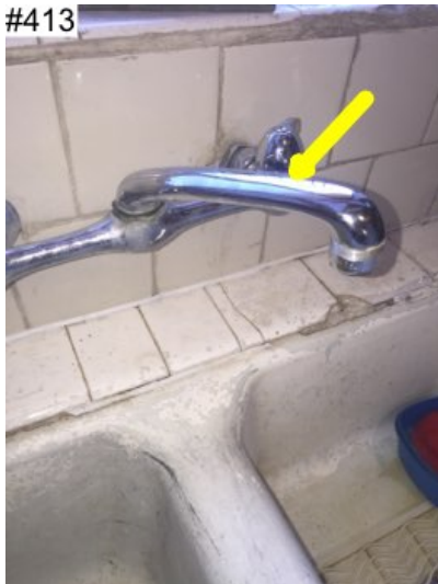
Faucet loose at base.
