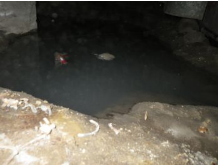
Standing water observed.
