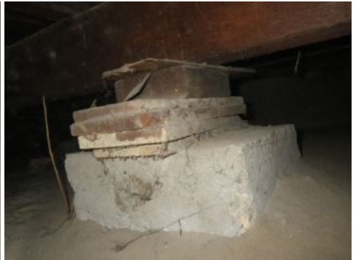
Improper materials used at various posts. see photos
