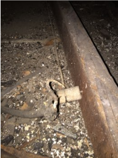
Live knob and tube wiring present.
