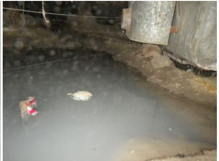
Standing water observed.
