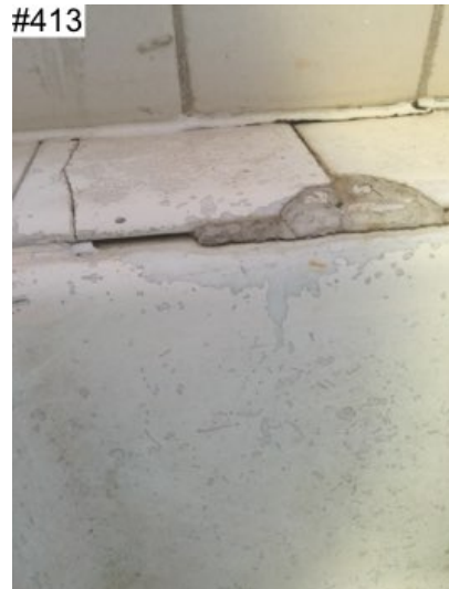
Suggest caulking as necessary.
