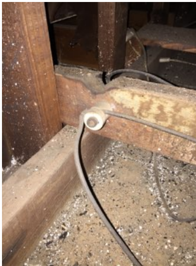
Live knob and tube wiring present.
