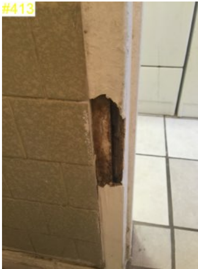
Damage to door frame
