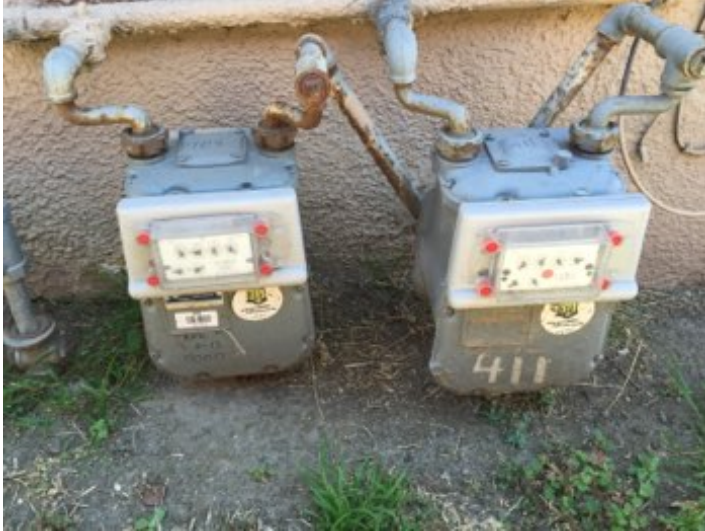
Meter located at exterior. All gas appliances have cut-off valves in line at each unit. No gas odors detected.
