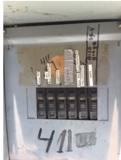
All of the circuit breakers appeared serviceable.
