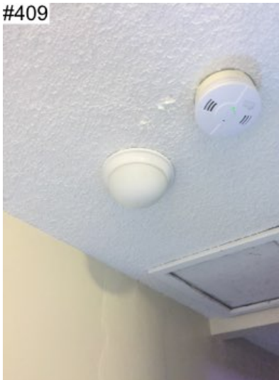
Light in hallway does not operate. Check lightbulb
