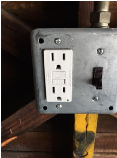
GFCI in place and operational
