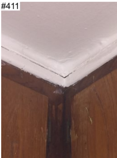
Noted cabinet(s) separating at the ceiling. Recommend having a qualified contractor re-fasten the cabinets. #411
